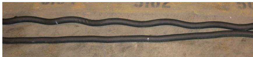
Figure 1: Cables that have the corkscrew condition
