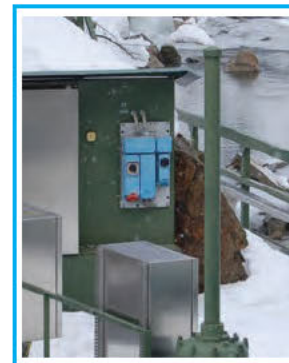
Hydroelectric power plant
